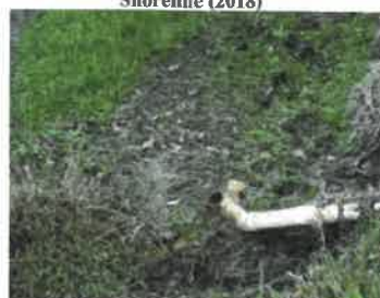
Inflow pipe from pump (2018)
