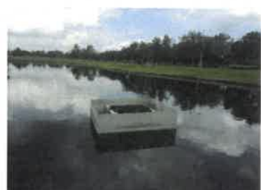
Control Structure after Hurricane Irma (09/2017)
