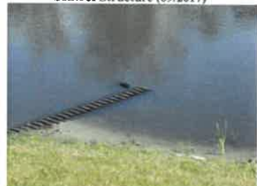
Exposed inflow pipe (2018)
