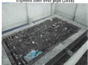
Control Structure with debris on grate (2018)
