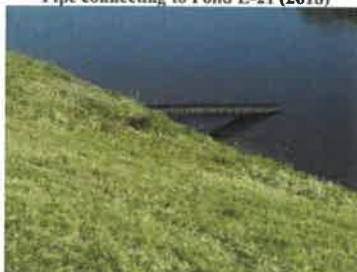
Exposed inflow pipe from golf course (2018)
