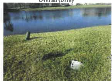
Broken reclaimed water lid (2018)
