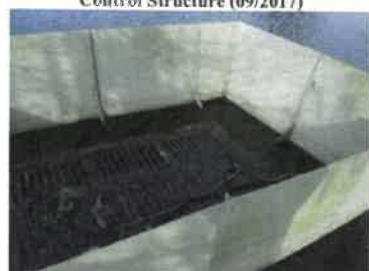
Control Structure with debris (2018)
