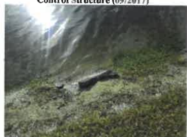
Inflow pipe end section (2018)
