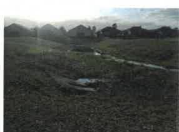
Inflow pipe from spreader swale capturing flow from residential area into beginning of swale into Pond E-18 (2018)
