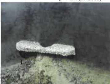
Inflow pipe end section (2018)
