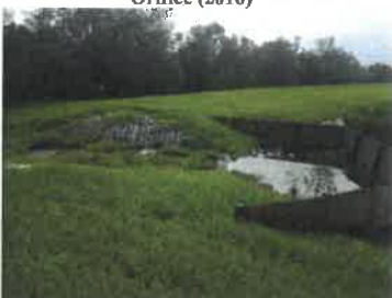
Overflow weir and Skimmer (09/2017)
