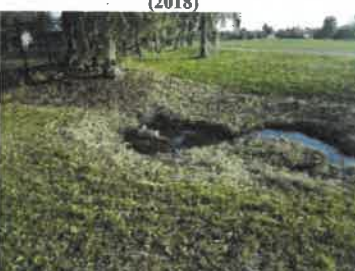
Spreader swale and inflow pipe from residential area (2018)
