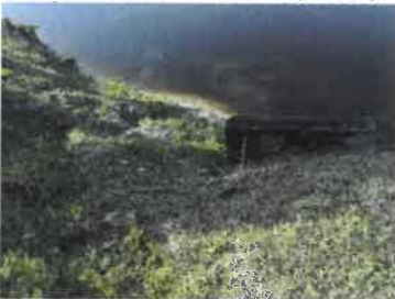
Shoreline erosion and inflow pipe end section (2018)
