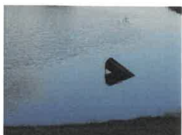
Exposed Inflow pipe (2018)
