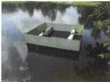
Control Structure after Hurricane Irma (09/2017)
