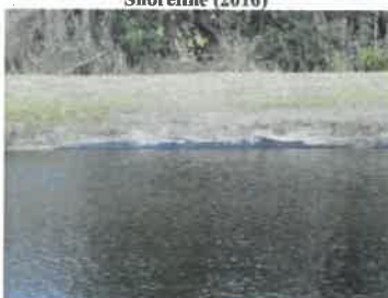
Shoreline erosion with pond slope protection exposed (2018)
