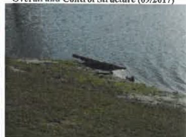
Inflow pipe end section (2018)
