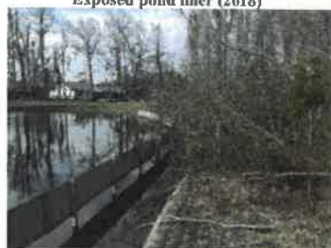
Weir and skimmer with overgrown trees (2018)
