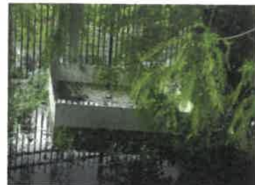
Control Structure showing debris (09/2017)
