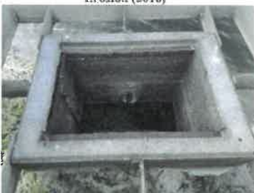
Control Structure missing grate (2018)
