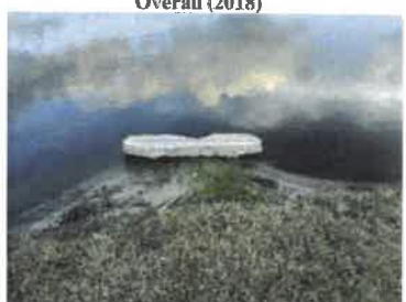
Inflow pipe end section (2018)
