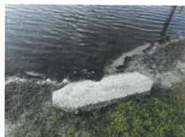
Minor Erosion around MES (2018)
