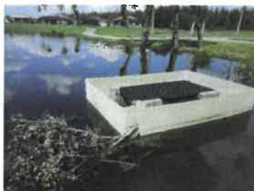
Control Structure with debris floating (09/2017)
