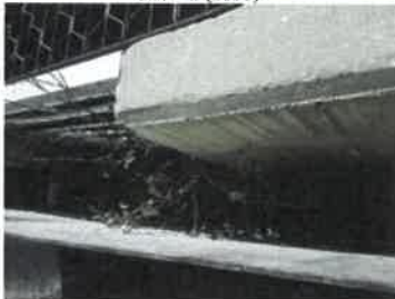
Nuisance vegetation inside control structure (2018)
