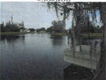
Shoreline erosion next to Control Structure (2018)
