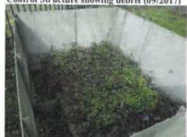
Control Structure Grate covered with debris and nuisance vegetation (2018)
