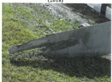
Damaged corner of skimmer (2018)
