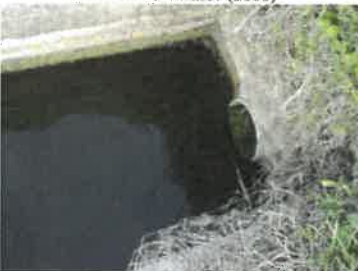
Orifice with missing stand pipe (2018)
