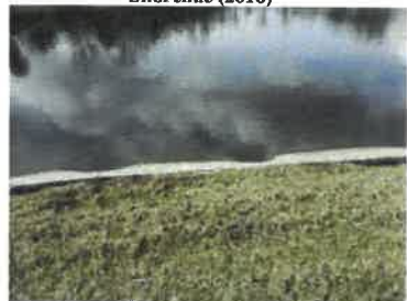
Connecting pipes end sections (2018)
