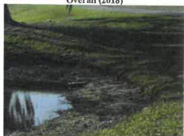
Exposed inflow pipe from golf course (2018)
