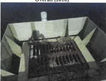
Minor debris on grate (2018)
