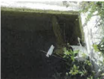
Orifice with debris blocking entrance (2018)
