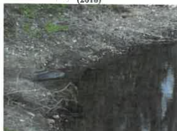
Exposed pond liner (2018)
