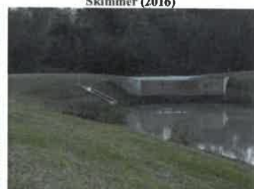
Overflow weir and skimmer (2018)
