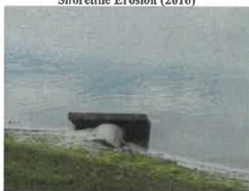
Inflow pipe end section (2018)
