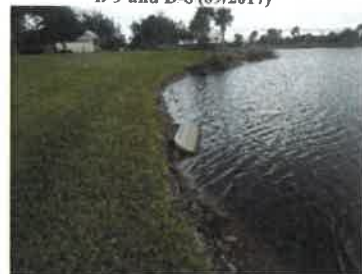
Inflow pipe end section (2018)
