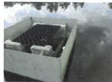
Control Structure after Hurricane Irma (09/2017)
