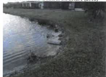
Shoreline and exposed inflow pipe (2018)
