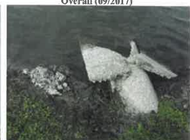
Damaged inflow pipe end section (2018)
