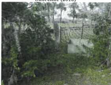
Control Structure surrounded by nuisance vegetation (2018)
