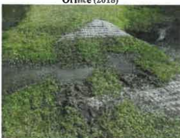
Weir with overgrown plants (2018)
