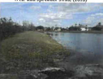
Damaged weir and shoreline (2018)
