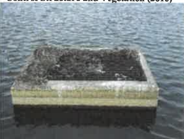
Control Structure with debris on grate (2018)
