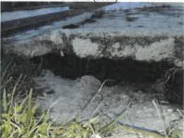
Erosion damage to side of weir (2018)
