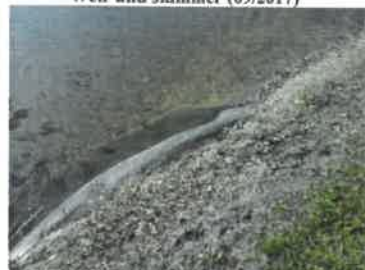
Exposed pond liner (2018)
