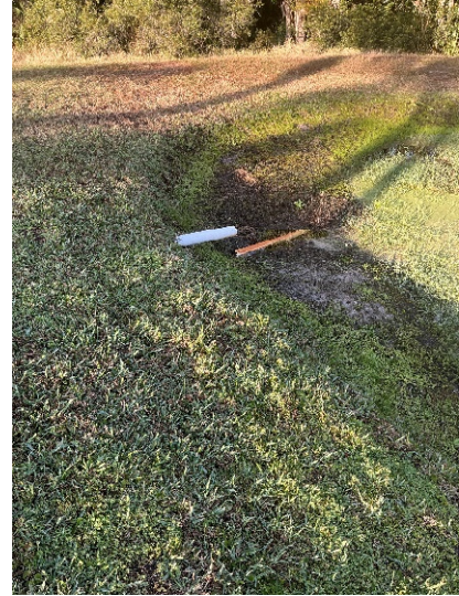
PVC pipe appears to be broken.
