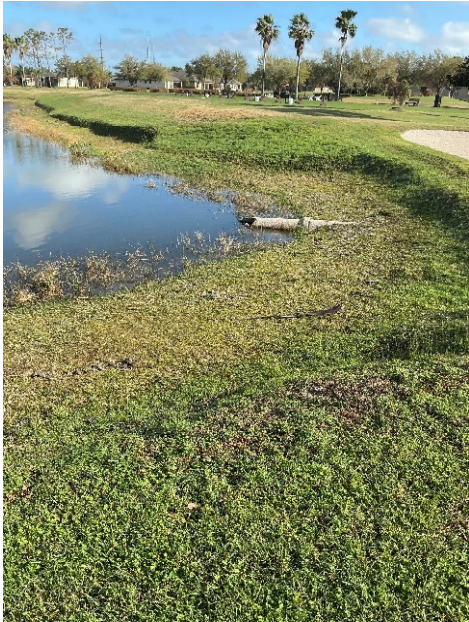
RCP pipe appears to function properly but is broken/damaged.
