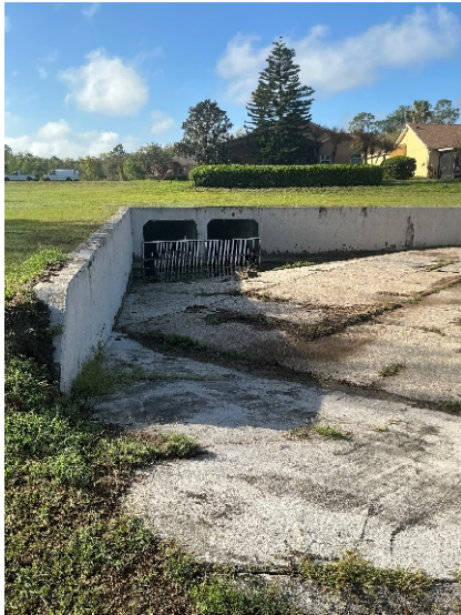
Some gate pieces are broken in front of the culvert. This does not affect fuction of the structure.
