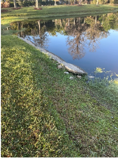
Submerged MES appears to be slightly damaged.
