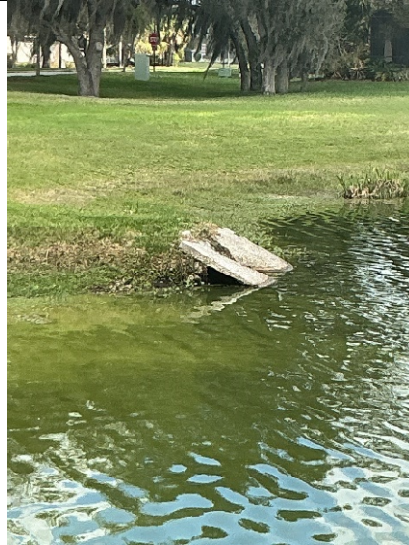
MES appears to function properly but is slightly damaged.
