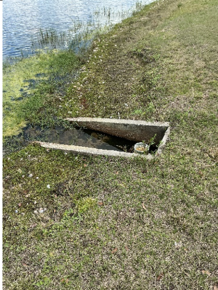
MES is good working order. Algae noted around and inside structure.
