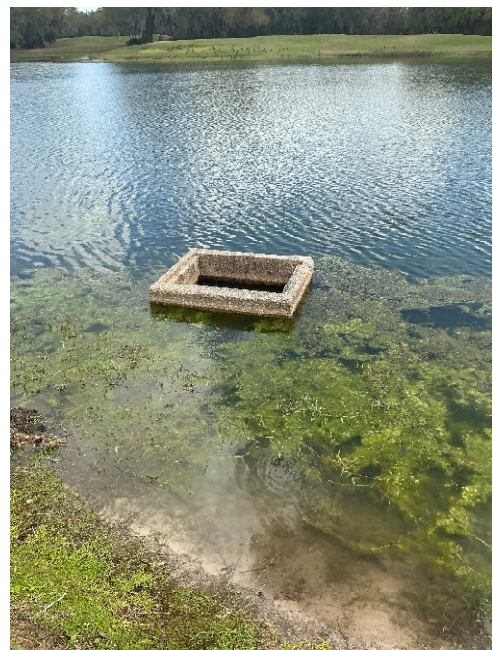
Control structure appears to be in good working order and functions properly. Algae surrounding it.
