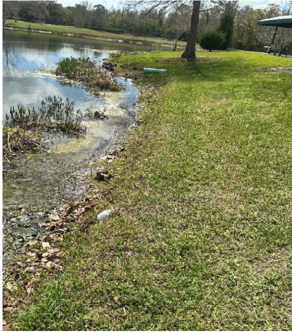
Another exposed PVC pipe (green) that is not flush with bank and could pose a tripping hazard.
