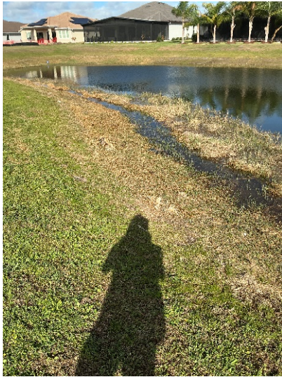
Corrugated pipe is broken/damaged. Bare slopes along pond bank.
