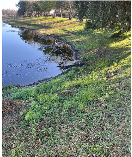
RCP pipe flowing into pond appears to function properly but is broken/damaged. Slight algae growth around pond perimeter.
