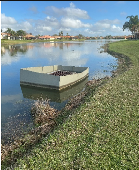
Control structure appears to function properly but is slightly warped around the edges.
